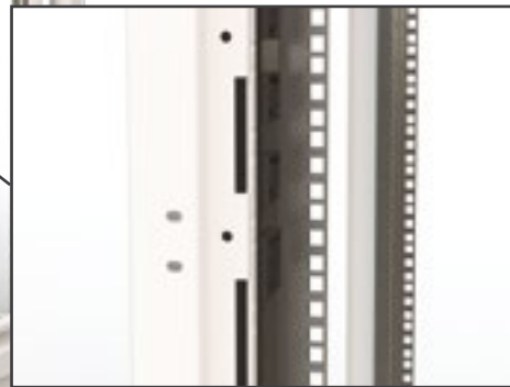
Typical position of vertical (0U) PDU in the rear side of the rack
